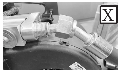
Improperly Seated O-ring Land
