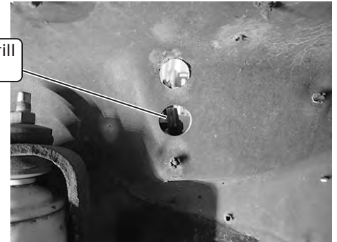
Wheel Well Side
